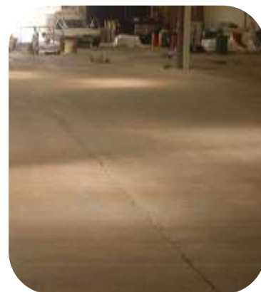
Concrete surface primed using Resichem 503 SPEP prior to application of Resichem 501 CRSG
